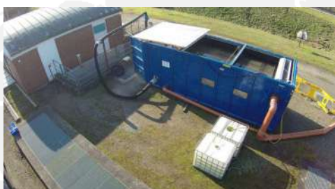
Lamella settler container solution at CSO facility
